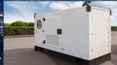
HARDWARE: Power Generator SOFTWARE: Remote management system
