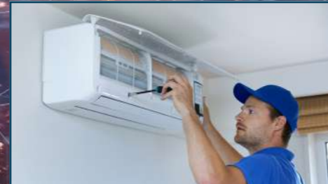
HARDWARE: Air conditioning unit SOFTWARE: Building management system
